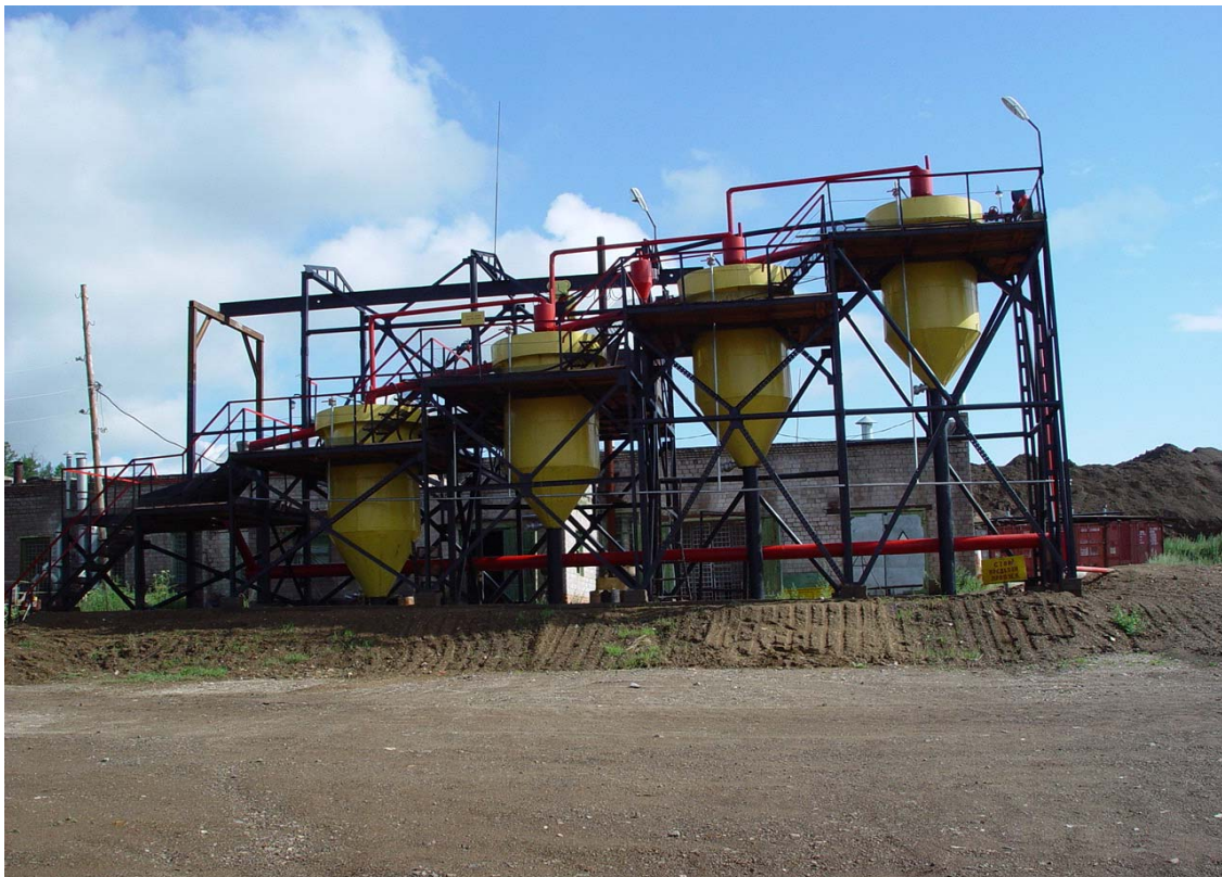
Fig. 49. General view of gold precipitation unit on activated carbon
