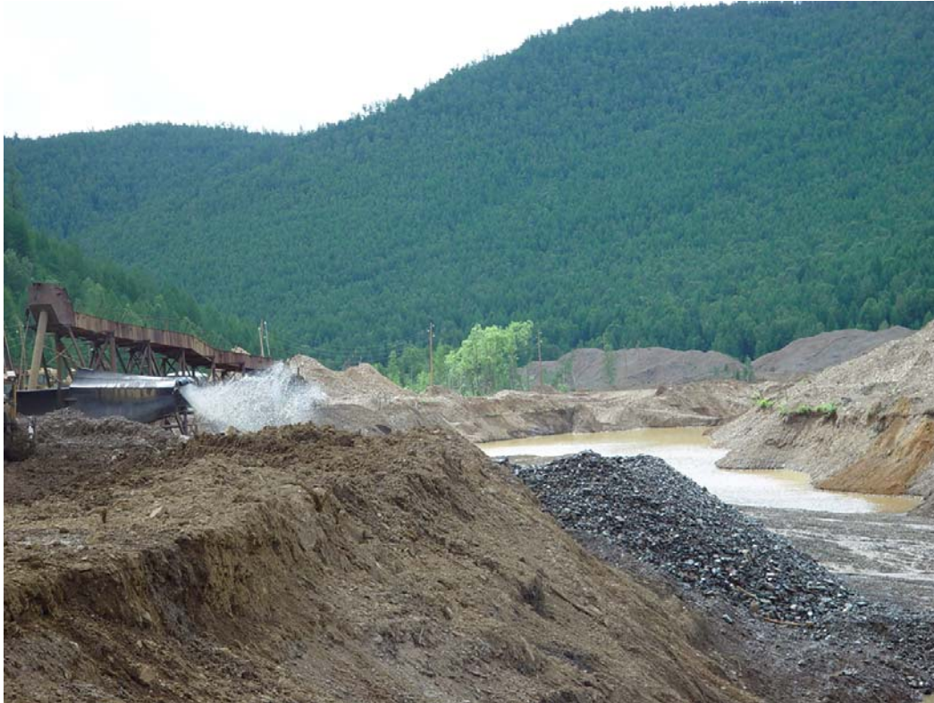
Fig. 25. Layout of overburdens and «sands» at gold field exploration on river Andat
