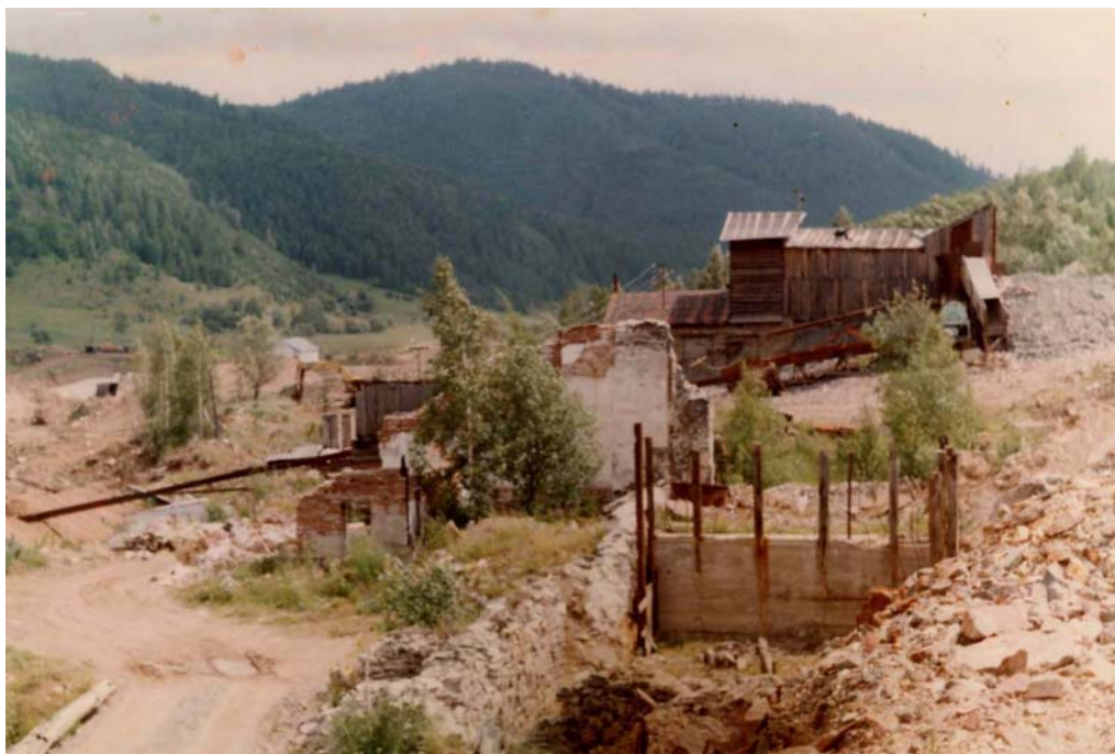
Fig. 29. Balakhchino gold field. Destroyed concentration plant. At the background one can see a waste treatment unit
