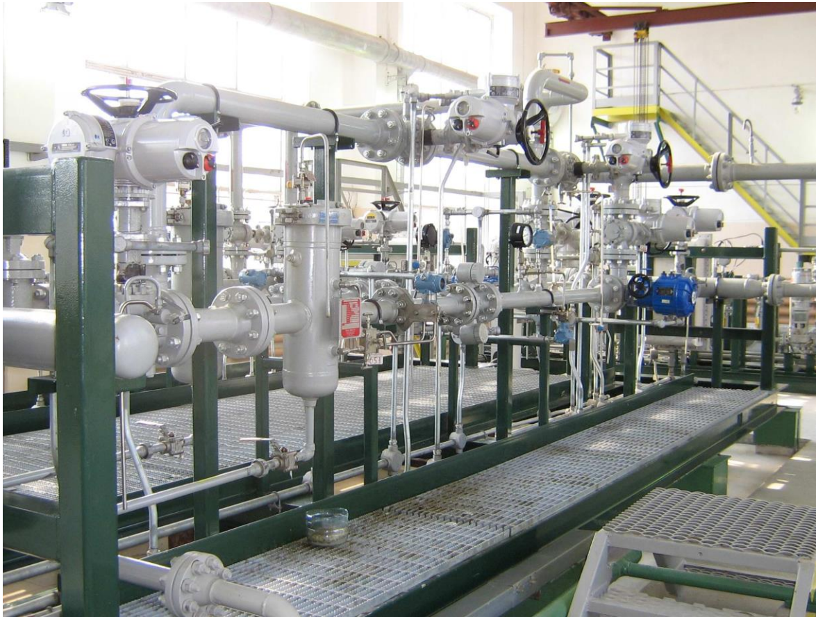
Fig. 4.15. Illustration of measurement system unit FMC Energy Systems, USA
