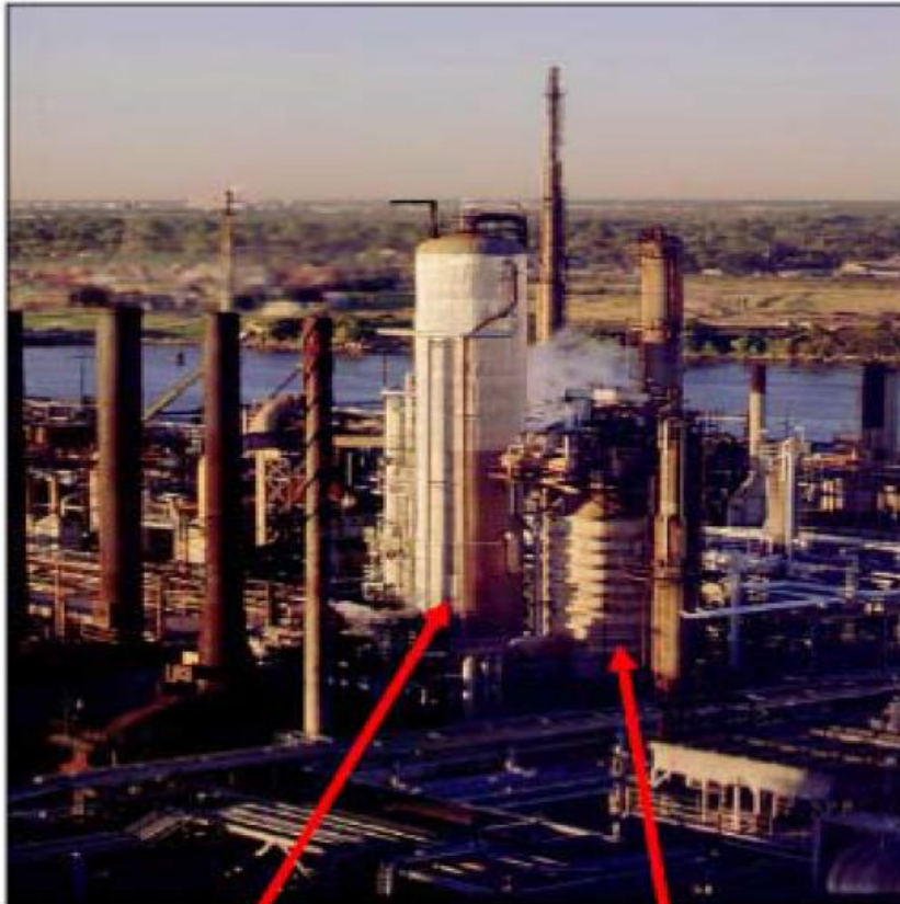
Crude Atmospheric Tower
