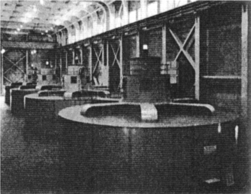
FIGURE 8.1 Four 100 MVA, 13.8 kV vertical-shaft hydrogenerators. The hydraulic turbines (not shown) are located on the floor below. (Courtesy of Seattle City Light.)
