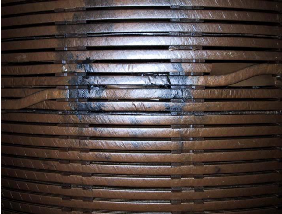
Figure 5.26 Damage to the HV winding of phase W as seen after opening of the transformer
